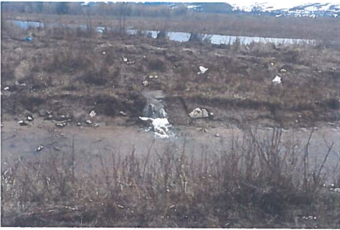
The Smiths Fork River was eroding the Whites Water Ditch away through active beaver holes.
