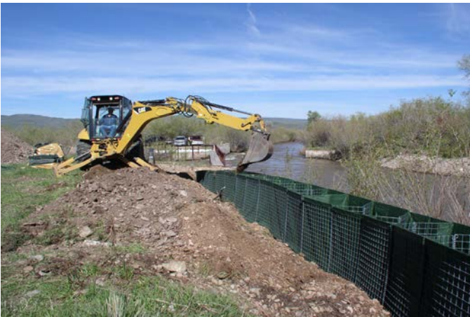
Hesco barriers were placed on the east dike of the tri-diversion structure to prevent a major washout.
