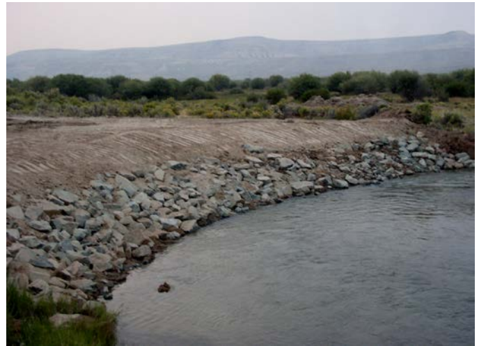
Rock rip-rap was placed on the north side of LaBarge Creek to stop bank erosion.
