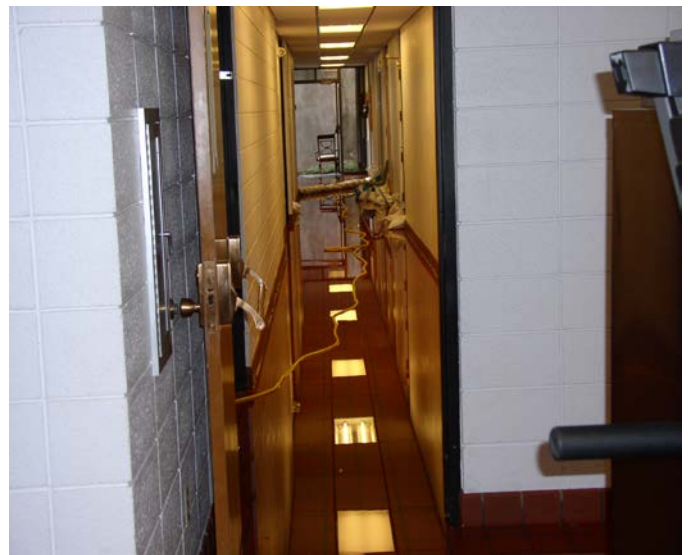
The Cokeville Town Hall's basement had severe ground water damage this past spring.
