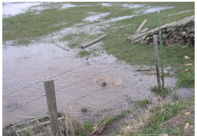
A hole in the north dike on the Smiths Fork River threatened several homes and U.S. Highway 30.
